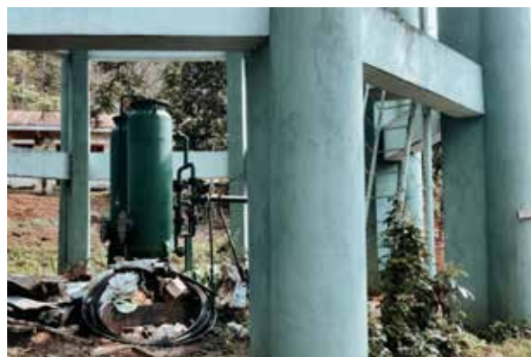
Water filtration unit at Medziphema, Nagaland
